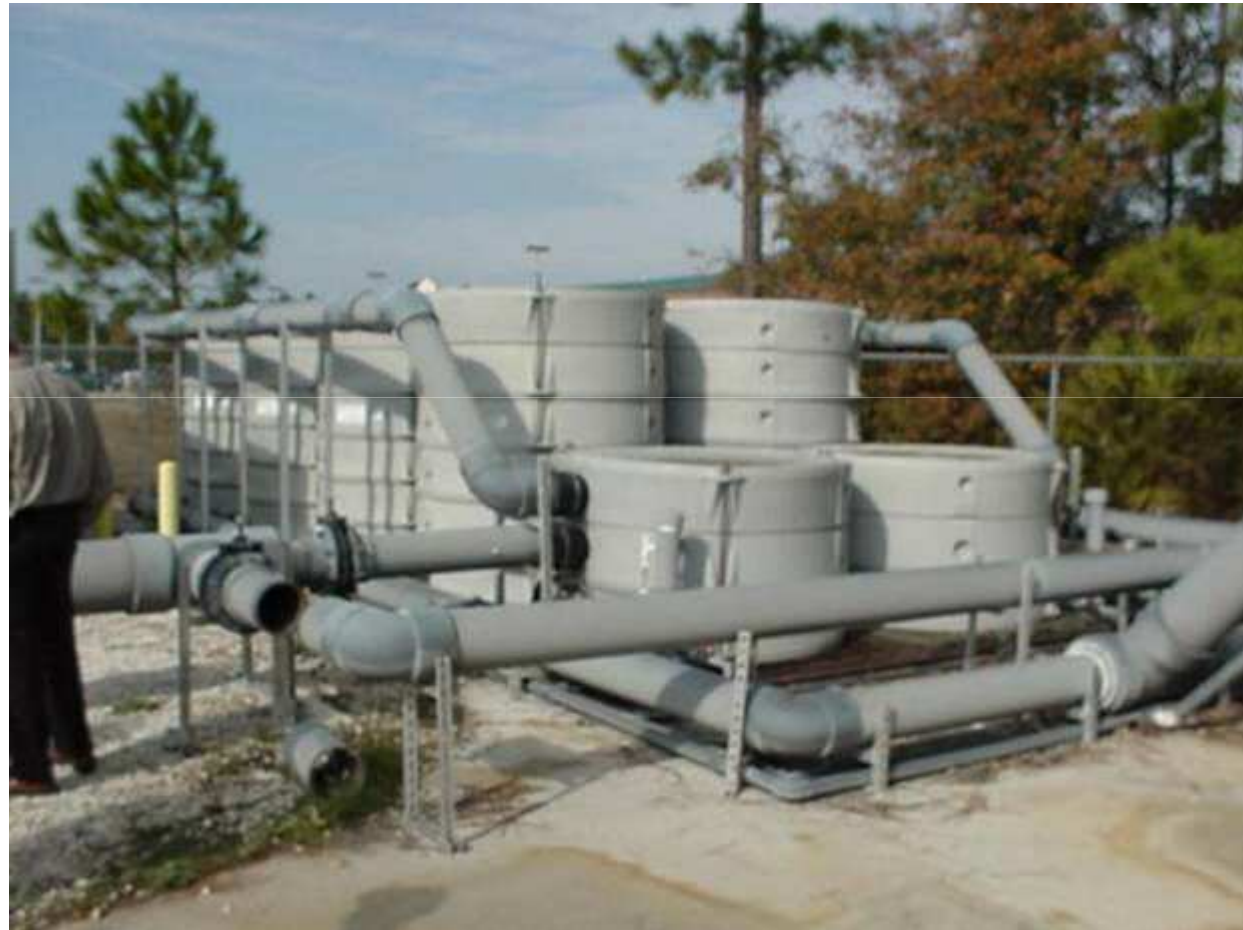
Abess Road Pump Station in Jacksonville, FL (JEA)
