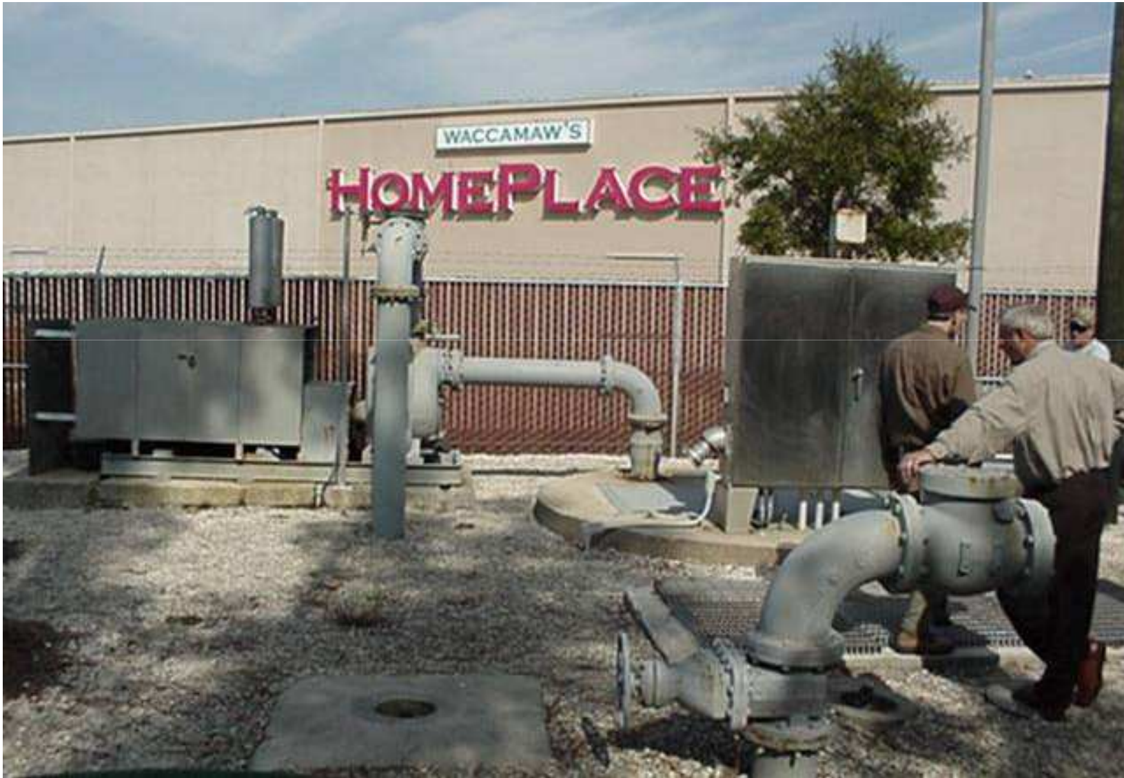
Iron sponge system on JEA collection system near mall
