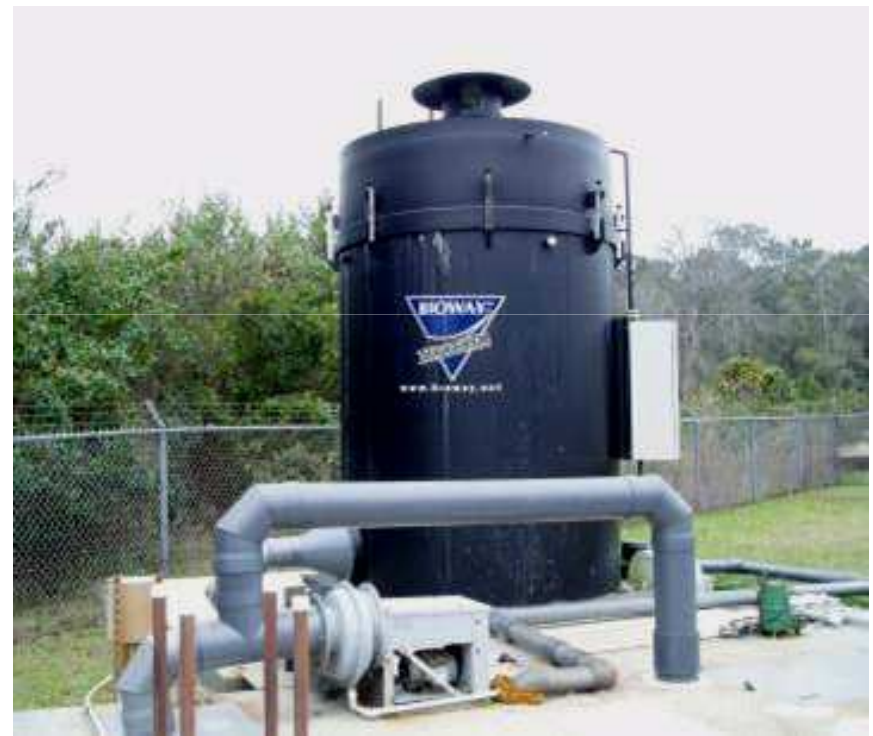
HDPE Bioway Zerochem® unit at Renne Drive Lift Station
