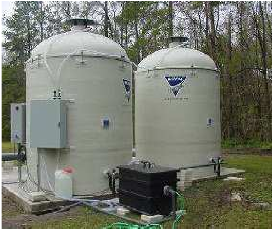
Fiberglass Bioway Zerochem® units at Lennox Avenue Lift Station
