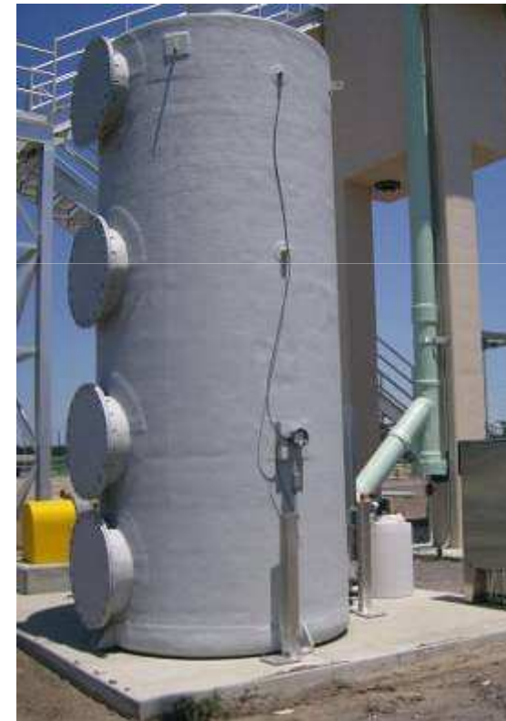
BIOREM installation in Lakeland, FL
